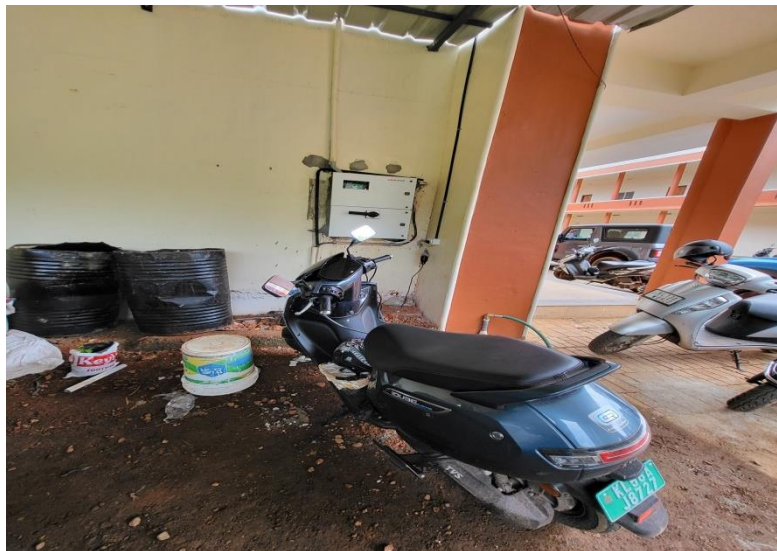
Figure 11 E-VEHICLE CHARGING FACILITY
